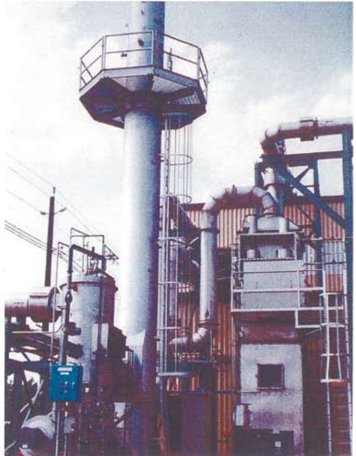
Wet Electrostatic Precipitator and Exhaust Gas Reheater at Somerset-Raritan Valley Sewerage Authority*, Bridgewater, NJ.
